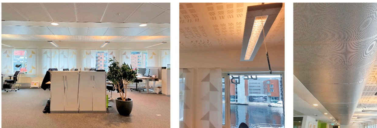
Figure 3. (Left): desk arrangement in a typical landscape layout; (Centre): daylight sensor for the operation of the external shading; (Right): ceiling-mounted diffuse ventilation channel.
