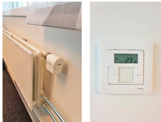
Figure 4. (Left): thermostat regulator mounted on a radiator. (Right): wall-mounted thermostat controller.
