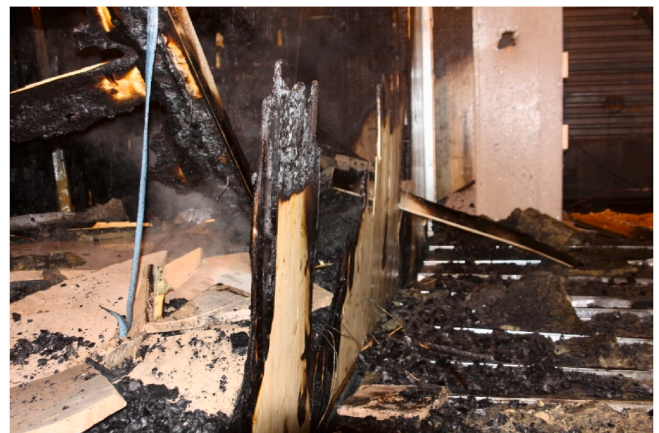
Fig. 18. Very little of the exposed CLT wall (Wall A) was remaining after the experiment. The light steel frame wall with stone wool insulation that was on the non-exposed side of the wall can be seen lying down to the right. The greyish pieces to the left are parts of the substrate layer from the collapsed ceiling. Photo by RISE Fire Research.
