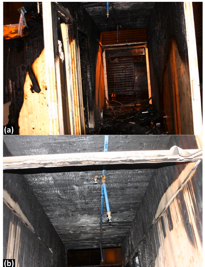
Fig. 16. (a) The corridor after the experiment. (b) The CLT ceiling and the upper walls of the corridor were heavily charred despite the activation of four sprinkler nozzles. The marks on the wall also show clearly which areas that were effectively protected by the water. Photos by RISE Fire Research.
