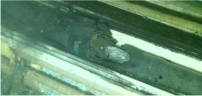
Figure 12: Fault located on piggyback cable.
