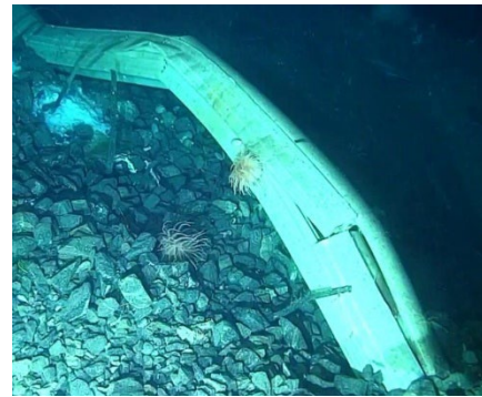
Figure 15: Piggyback cable protection snapped from flowline.
