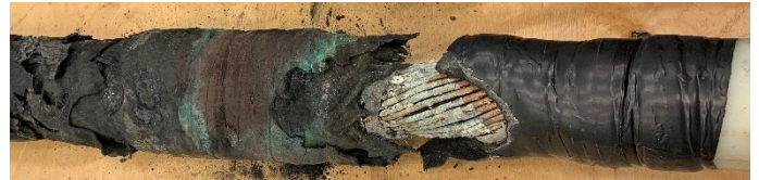
Figure 14: Dielectric fault of piggyback cable.
