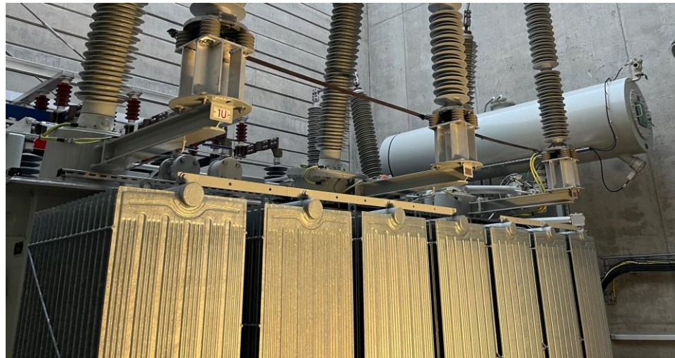
Figure 1. The three-phase 40 MVA power transformer in operation in the substation. The photo focuses on the auxiliary equipment: the radiators in the front, the HV-bushings and the surge arresters on the top and the oil expansion tank in the back.
