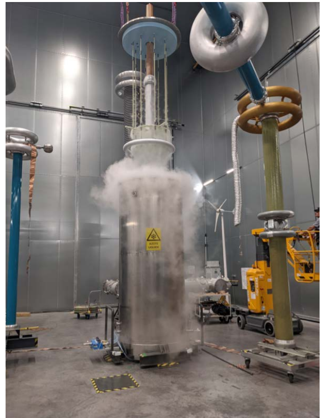
Fig. 6: High-voltage cryostat to be used for the demonstration tests of the RSFCL module
