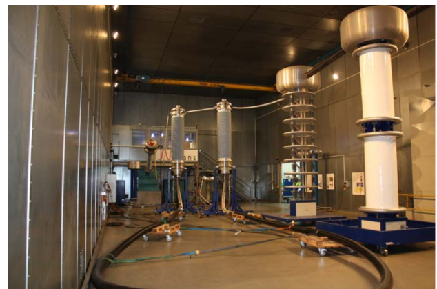
Fig. 3: Best Paths testing loop (cable and terminations) together with the 800 kV DC generator
