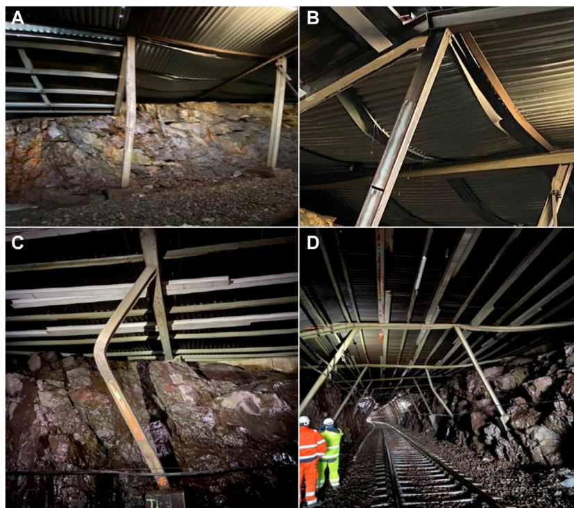
FIGURE 3 Failure of snow gallery 13A (A,B) and failure of snow gallery 9 (C,D) (Sas et al., 2021).
