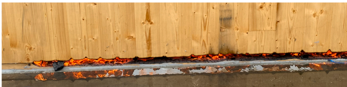
Fig. 31. The fire burned through the intersection between the back wall and the bottom plank at approximately 60 min. The image is taken at a later point when the gap had become larger. The lack of a fire sealant between the bottom plank and the CLT wall enabled this and highlights that connection details are crucial to fire safety.
