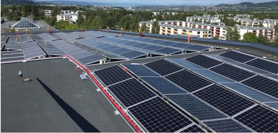
Figure 6. BAPV modules mounted on the roof at Heimdal Upper Secondary School [Source: Trøndelag County Council].
