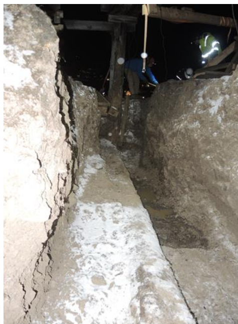
Figure 6. Reconstruction of foundation of cableway post Nr. 7, Line 5-6. Copyright: © Store Norske Spitsbergen Kulkompani.
