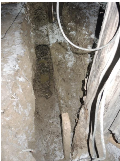
Figure 5. Reconstruction of foundation of cableway post Nr. 7, Line 5-6. Copyright: © Store Norske Spitsbergen Kulkompani.
