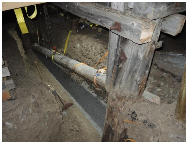
Figure 4. Reconstruction of foundation of cableway post Nr. 7, Line 5-6. Copyright: © Store Norske Spitsbergen Kulkompani.
