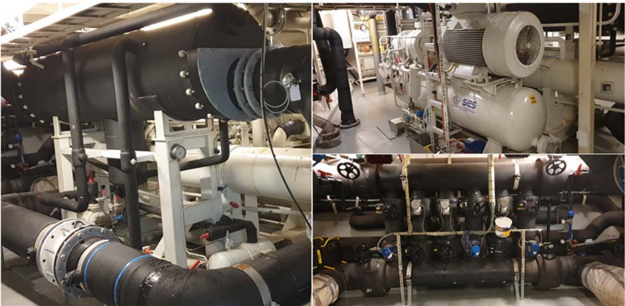
Figure 2: Pictures from machine room. Left: evaporator. Top right: Compressor package. Bottom right: Part of valve station for RSW system
