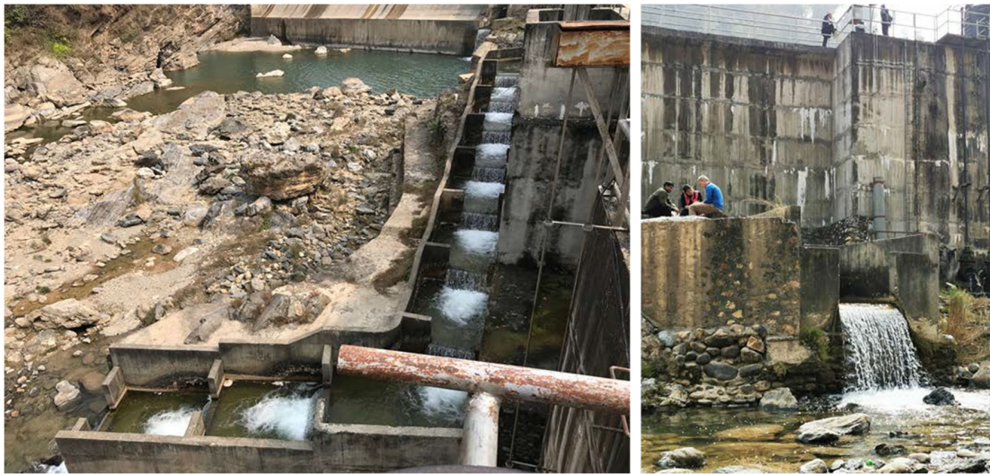
Figure 7. Pool type fish ladder at the Andhi Khola HPP (left) and entrance to the fish ladder (right).
