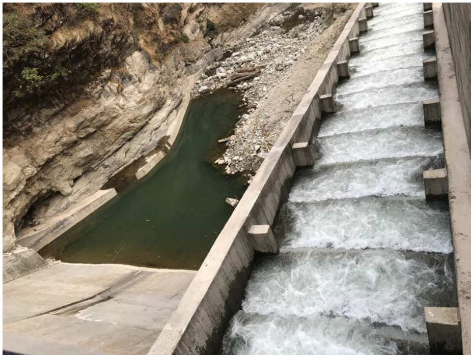
Figure 5. Vertical slot fish ladder at Upper Trishuli -3A HPP
