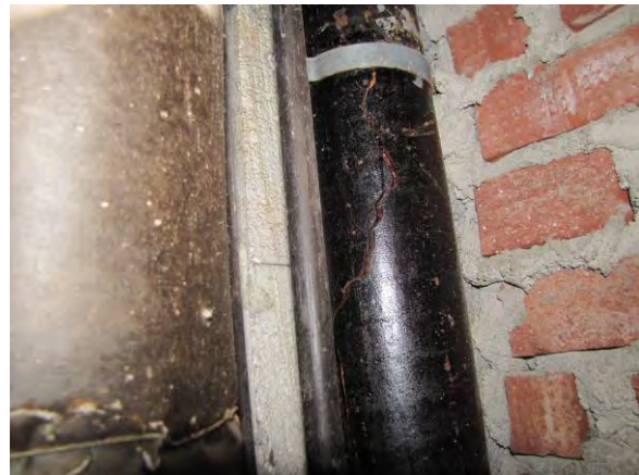
Figure 7. Various air leaks from drainpipes is a common cause for odour problems.
