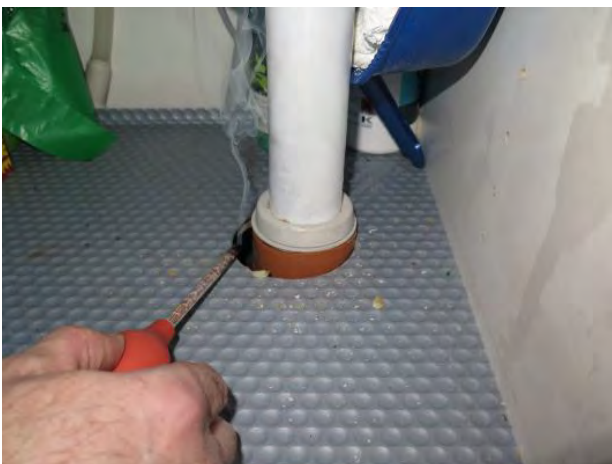
Figure 6. Air leakages transport odour from the source to other areas.
