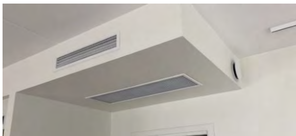
Figure 8: E-H0702 Fan coil
