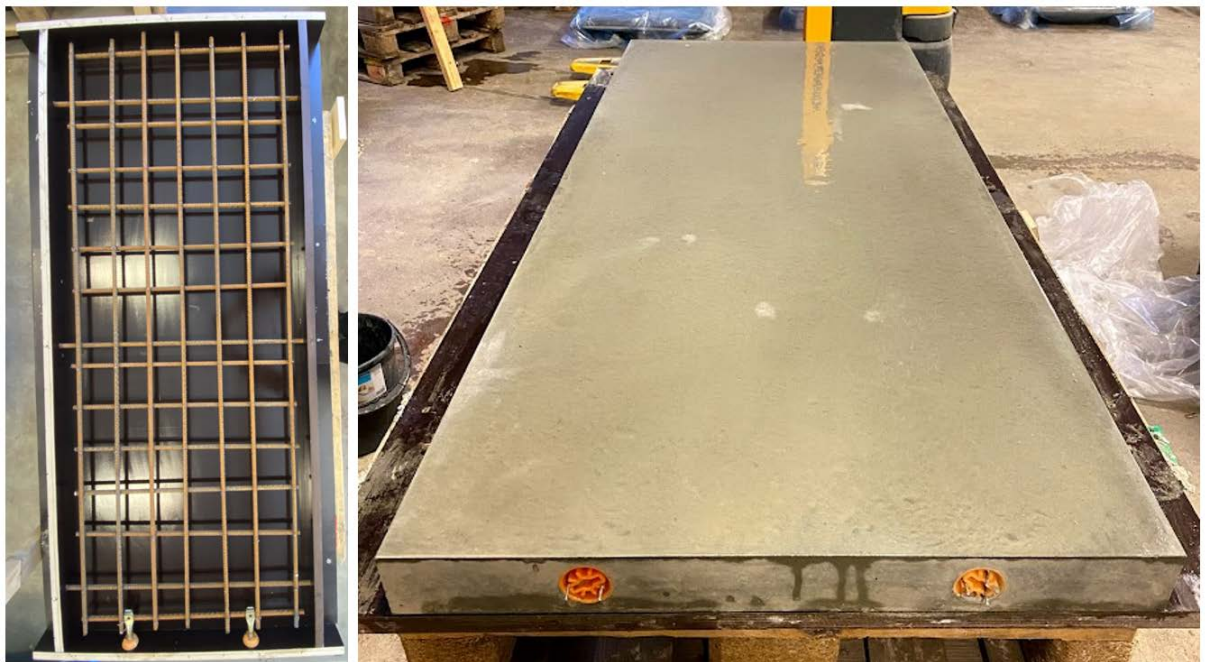
Figure 5.1: Formwork, reinforcement, and Vemo sleeves (left), a concrete segment straight after removing the formwork with the drying surface facing upwards (right).
