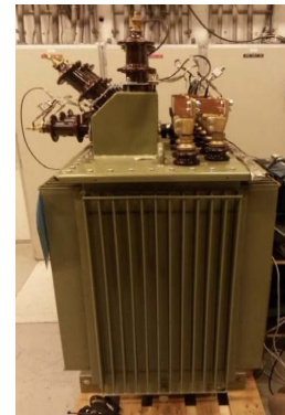
Fig. 2. Distribution transformer. Left: HV terminals; right: LV terminals.
