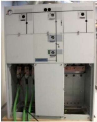
Fig. 2. Medium voltage test device. The enclosure corresponds to an SF 6 -filled 12/24 kV switchgear. The device was connected with the three phases on one side and the other side short circuited.
