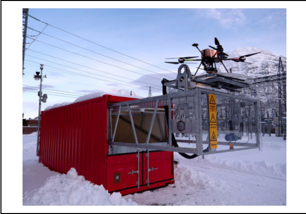
Figure 1. Drone and hangar at Aura substation, residing below the mountains. Photo by Thomas Negård.
