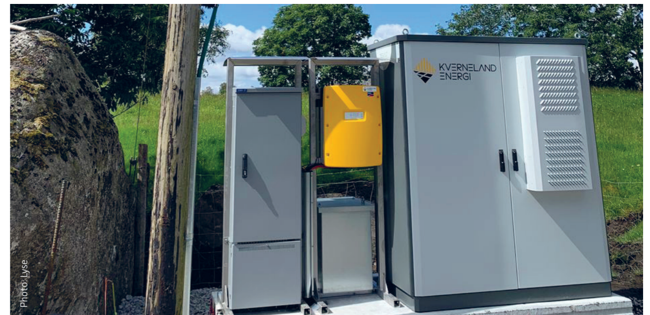
The system consists of an outdoor battery housing that provides voltage support to a small 230V overhead grid that supplies low voltage at certain periods.
