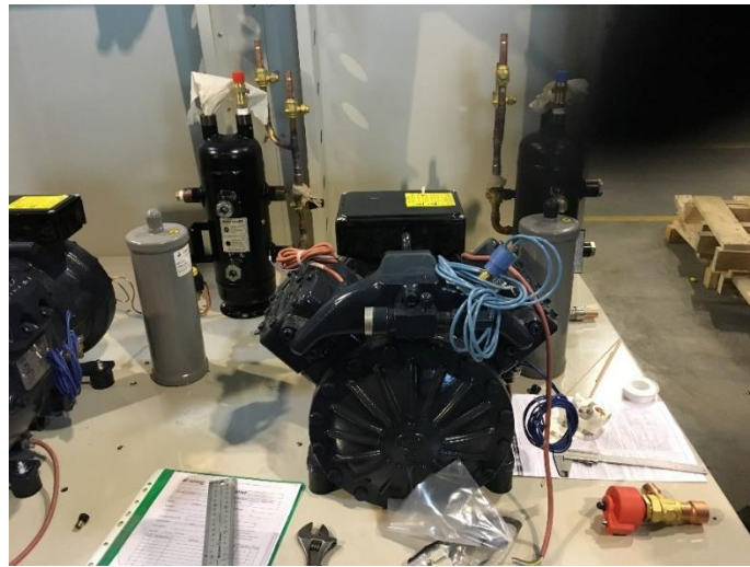
Figure 1: Installation of the modified R600 compressor for high temperature cycle
