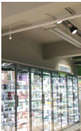
Figure 39. Air diffusers installed on the ceiling.
