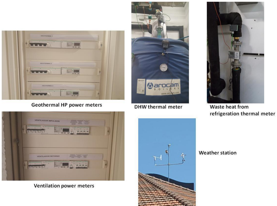
Figure 19. Real pictures of the meters inside the building and the weather stations on the roof
