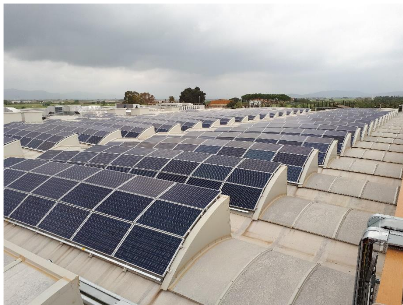
Figure 112. Photovoltaic system installed on a portion of the roof of Marema'
