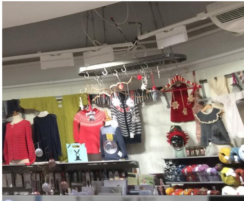
Figure 80. Application of the wallwasher in a retail shop in the demo case Trondheim.
