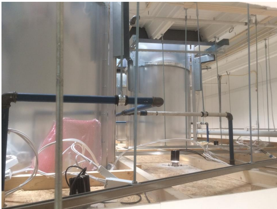
Figure 82. Picture of light tube installed between ceiling and roof
