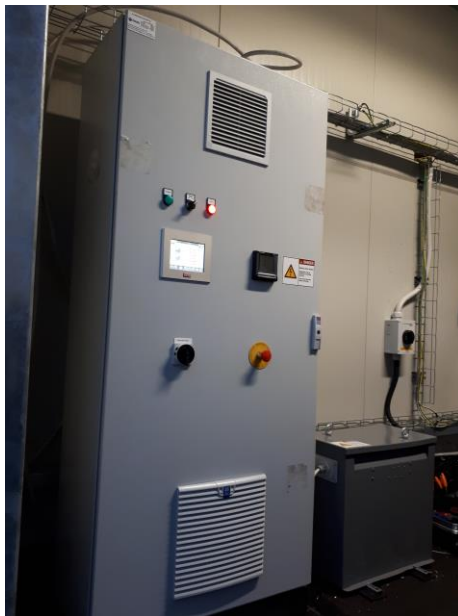
Figure 114. Bi-directional inverter cabinet for battery energy system installed in the technical room
