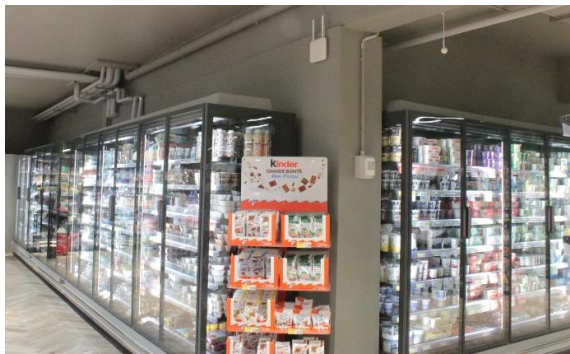
Figure 38. New refrigeration cabinets in the food store.
