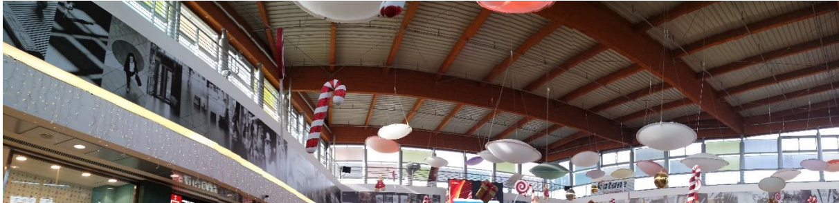
Figure 176. Stairwell shaft luminaries.
