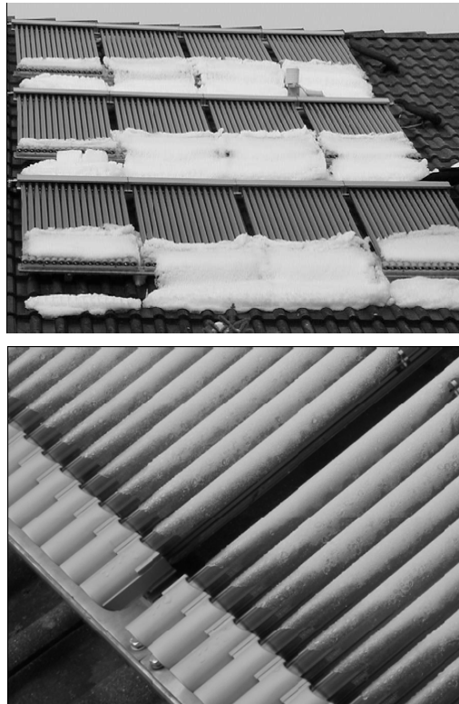
Figure 14. Snow (top photo) and frost formation (bottom photo) covering solar thermal panels (solar collectors) (Trinkl et al. [73]).
