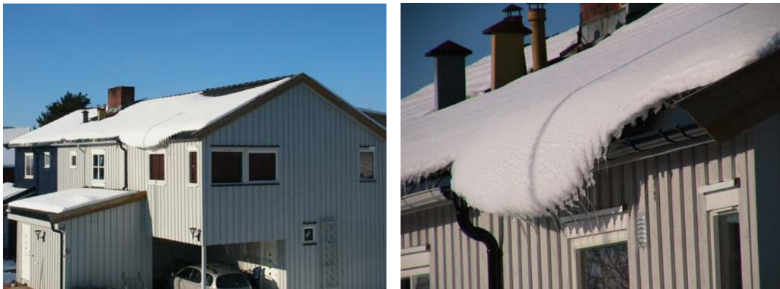
Figure 6. Right part of the roof of the above building was exchanged with smoother roof tiles, resulting in lower snow friction and a rather peculiar view from one of the windows. (Photo: SINTEF Building and Infrastructure).
