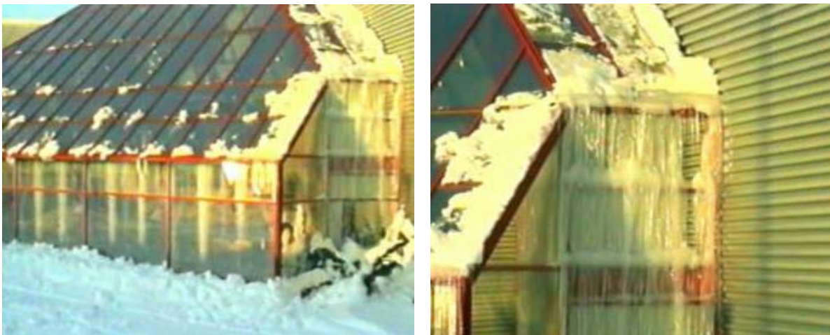
Figure 3. Large icicles covering the glass facade at a shopping centre (left) and close-up of the right part of the left photo, where the ice is completely covering this part of the glass facade (right). (Photo: SINTEF Building and Infrastructure).
