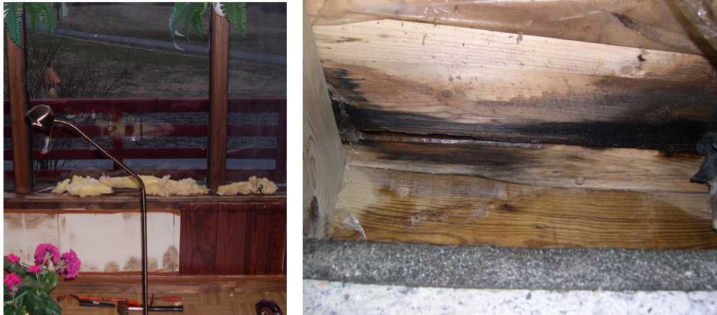
Figure 20. Large wood rot decay and fungi growth damages in a window and the construction below caused by moisture penetration during many years. The window had not been tested versus accelerated climate ageing and raintightness.
