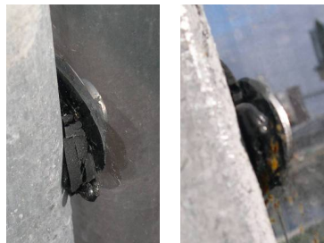
Figure 15. An example of a building damage case where the facade glass gaskets after short time did not withstand the climate strains.
