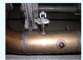
Sensor inserted in exhaust pipe.
