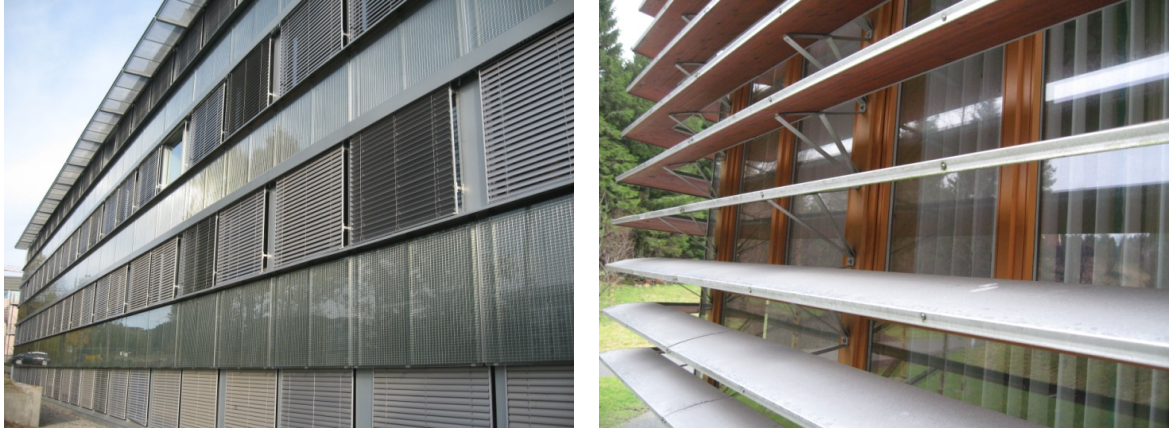
Figure 6.9: Example of external shading with automatically controlled venetian blinds on the left (Miljøsender Blindern) and fixed louvers on the right (Telenor Kokstad); Photos: SINTEF Byggforsk
