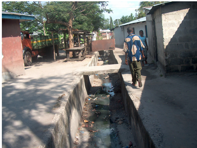
Fig. 2.17 Solid waste disposal in open drain
