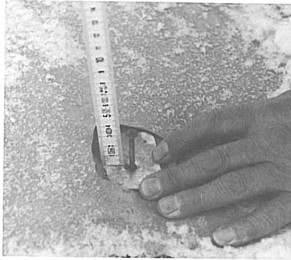
Photo 18 Roof III; screw backout
