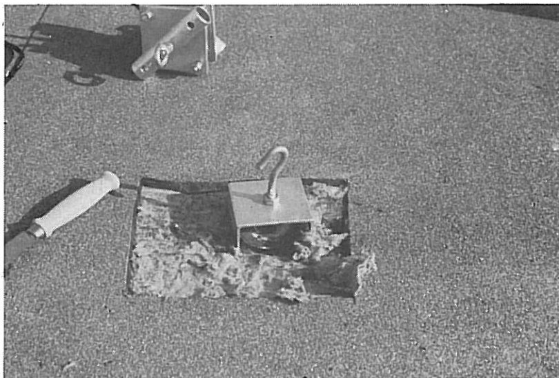
Photo 1. Membrane is cut open at fastener and shoe for pullout test is mounted.
