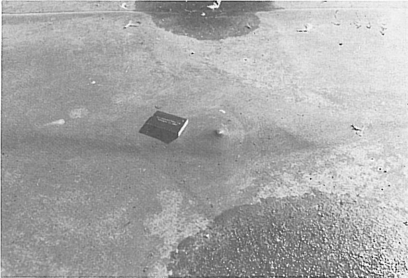
Photo 12. Example of loose screw mounted wrongly between ribs in steel deck. In time the membrane will be punctured.
