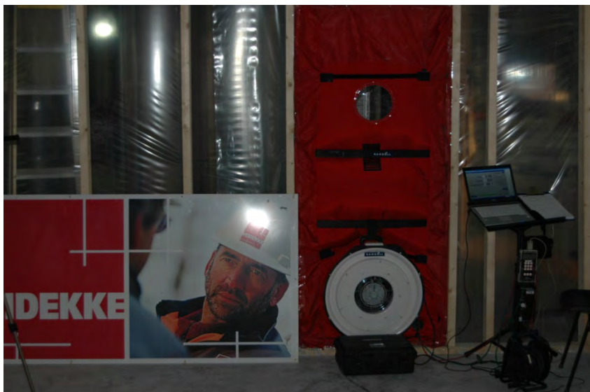
Figure 10 - preliminary air-pressure test of a part of the building with the usage of a Blower Door (ill. Rambøll Norge AS)
