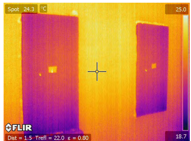
Two elements studied by IR thermography to investigate the influence of lattice girders on heat conduction.
