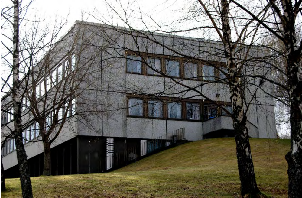
Figure 13 - Facade towards the North East of the existing building showing the prefab concrete elements (ill. Rambøll Norge AS)
