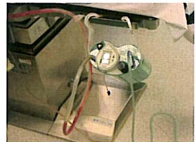
Air leakage system
