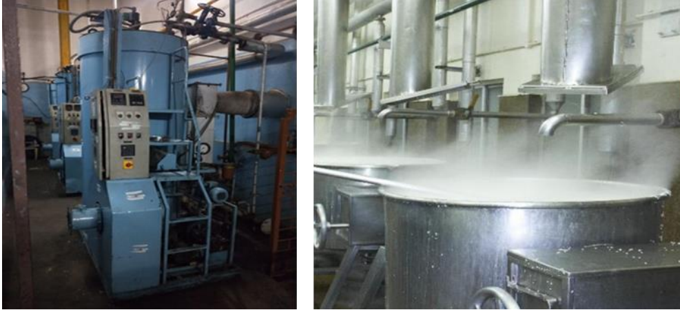
Figure 2-2: Steam boilers and cauldrons at Bengaluru kitchen
