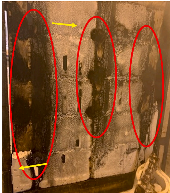
Fig. 22. Damage to the EPS insulation following Test 2 (a single layer of fire-retardant chipboard, test duration: 10 min).
