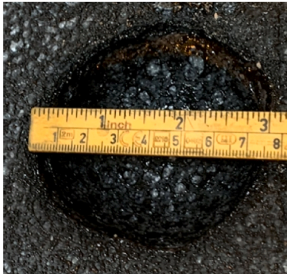
Fig. 30. Extent of damage to underlying EPS substrate behind 28 mm hole in the covering. Fire-retardant EPS substrate experienced an extent of damage of approximately 75 mm.
