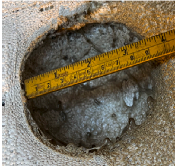
Fig. 29. Extent of damage to underlying EPS substrate behind 28 mm hole in the covering. Standard EPS substrate experienced an extent of damage of approximately 90 mm.
