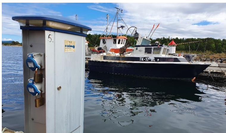
Figure 2 AC industrial sockets installed at a marina
