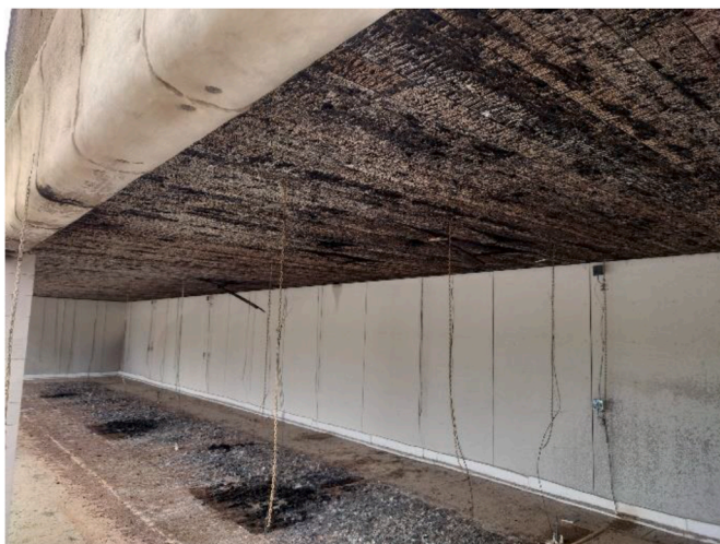
Fig. 14. Compartment after burn-out of the wood crib. No gypsum boards had fallen down, and the wood crib was completely consumed.
