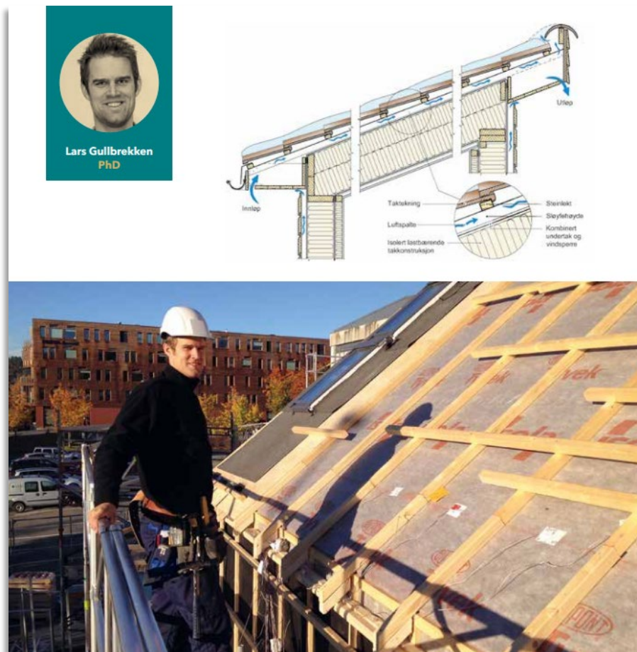
Figure 18: Lars Gullbrekken performed experiments at the roof of The ZEB Test Cell Laboratory
