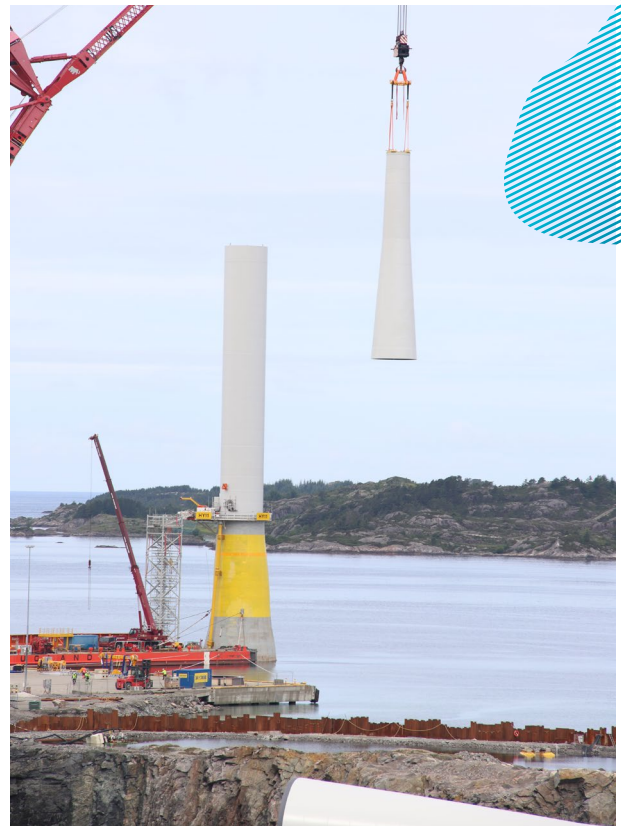
⚡ A floating wind turbine's tower is being assembled at Gulen, in Western Norway.
