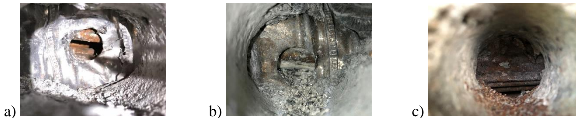
Figure 4 – Grouting and tendon status: a) Missing grout and three of the tendons are broken, b) An injected duct and c) Missing grout and the tendons are corroded.
