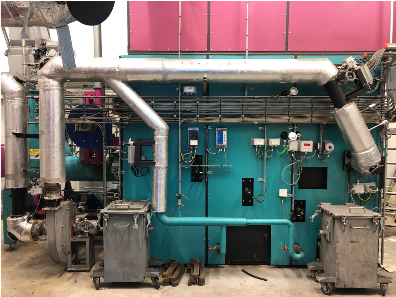
Figure 2.2 Tiller pilot plant 250 kW multifuel (coal/biomass) burner
