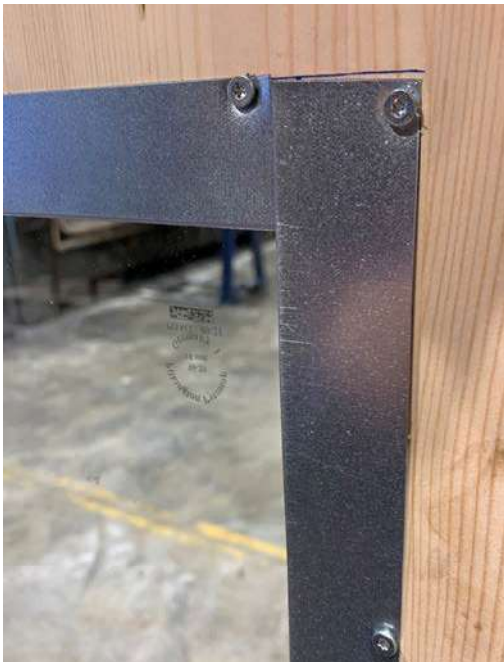
Figure 3-4 Detail for mounting of 30 mm steel frame. The steel frame can be hidden behind wooden battens for aesthetic reasons.
