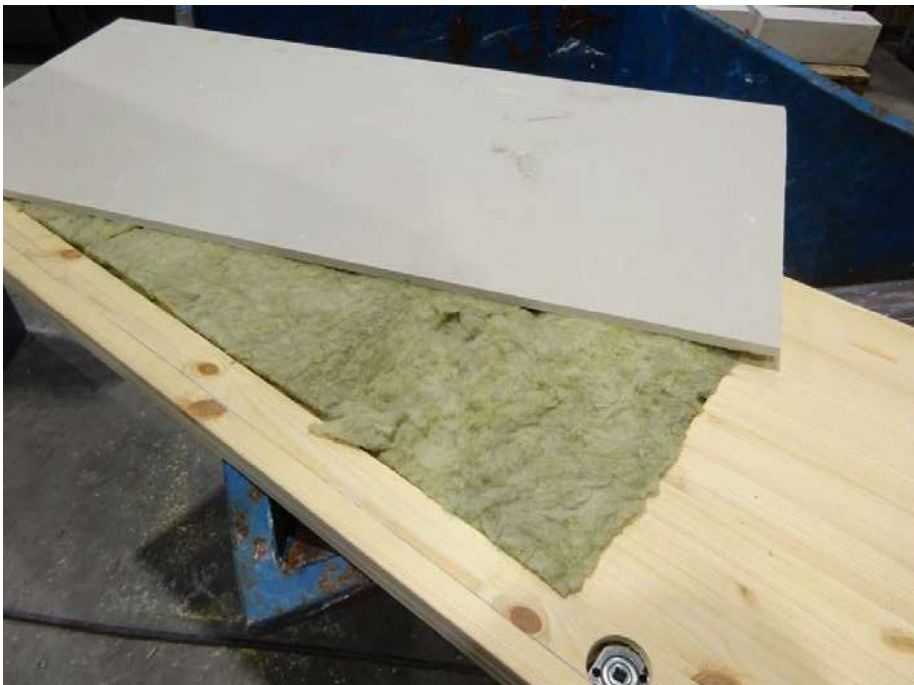
Figure 3-9 Detail for mounting of stone wool and robust gypsum board on wood panel
