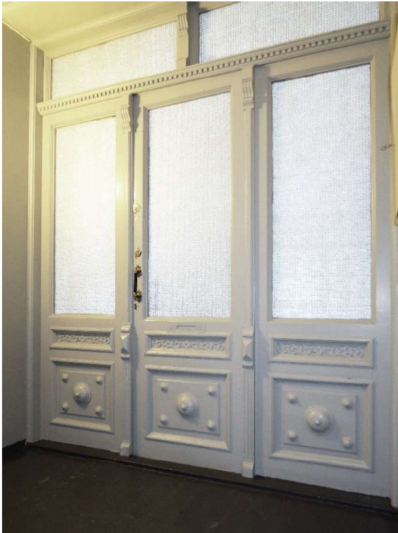
Figure 2-1 typical original stairwell door in older brick apartment house of cultural heritage value. [Photo credit: Jømna]
