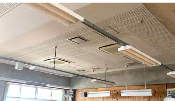
Figure 4. Two AC units and a ventilator on the ceiling
