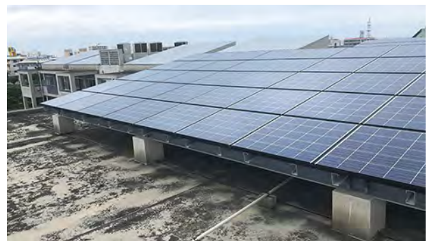
Figure 14. PV arrays on the rooftop
