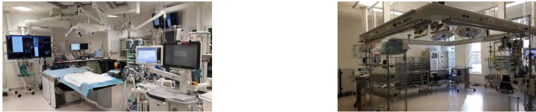
Figure 1. Mixing (left) and laminar air flow (right) ventilation solution OR in X hospital
