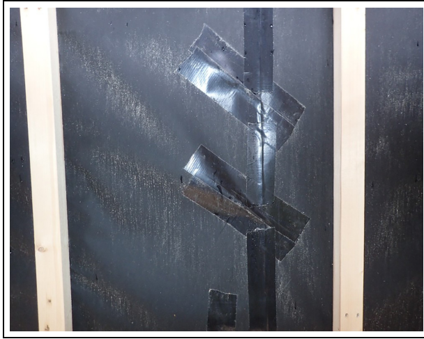
Figure 1. A taped joint in the wind barrier of the case building. Tape is also used to repair minor tears in the wind barrier.
