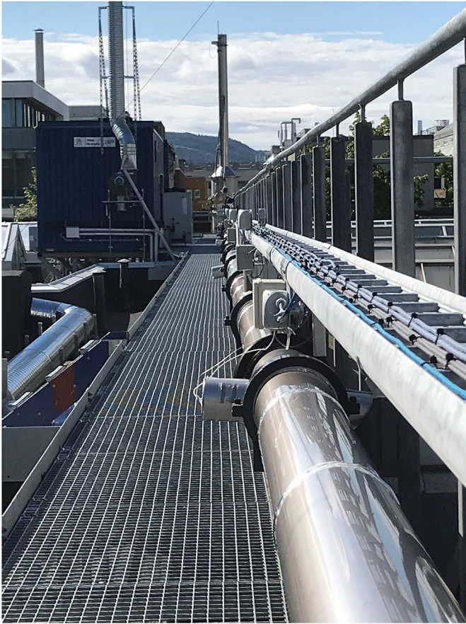
Fig. 2. The ECCSEL depressurization tube. The CO 2 is vented through the stack in the background. The container at the left contains support equipment.
