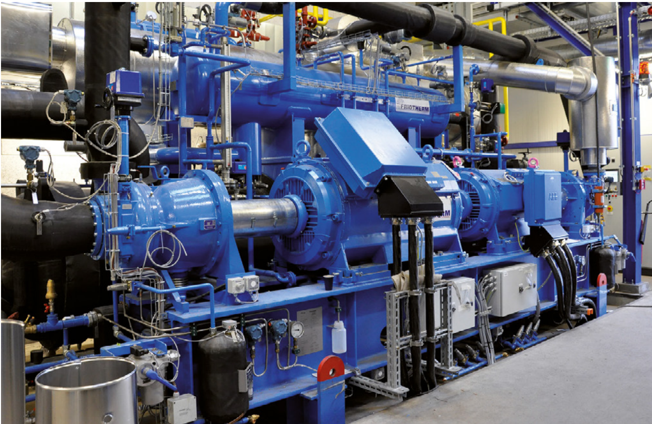
Figure 7: Heat pump installed at the Marienhütte steel and rolling mill Source: 17
