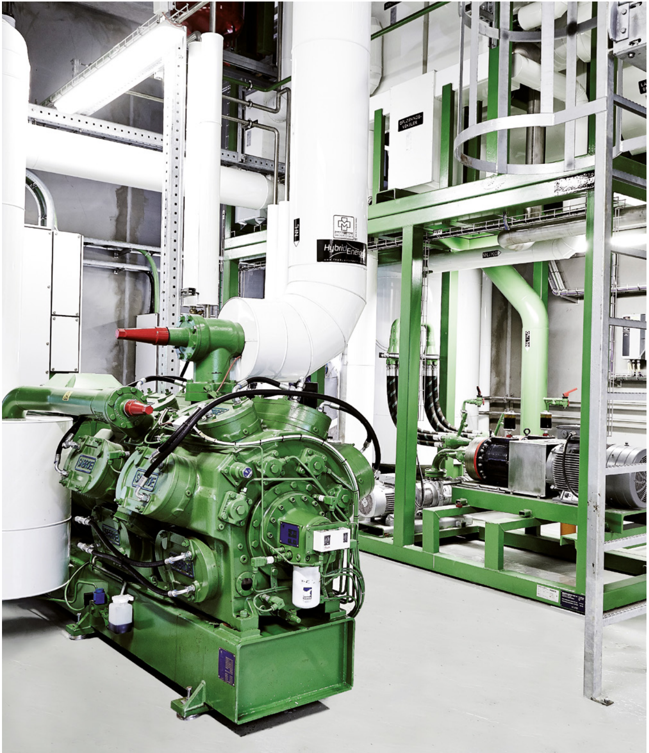
Figure 6: Heat pump installation at Arla Videbæk dairy
