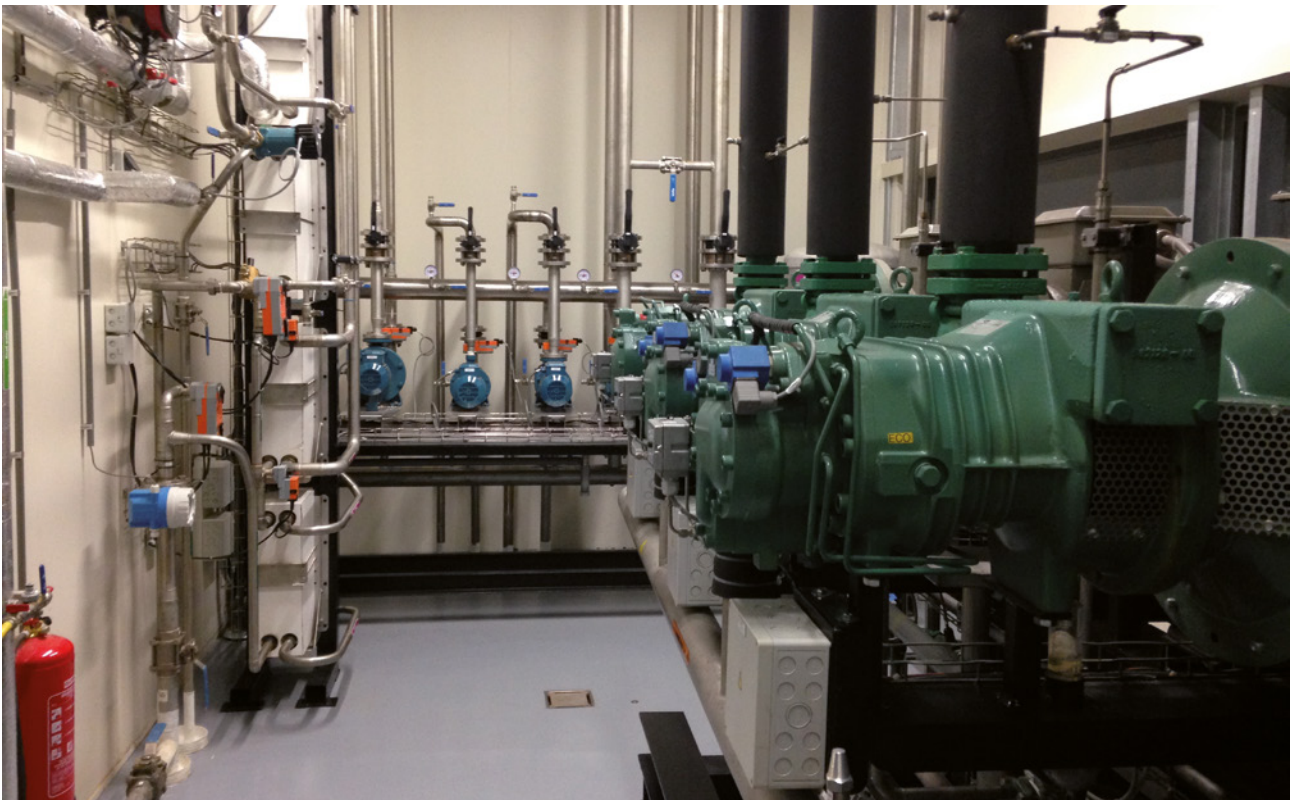
Figure 5: Heat pump installation at Hutten slaughterhouse
