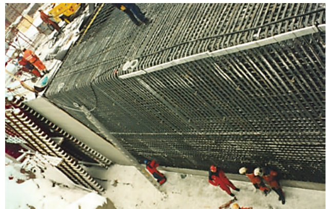
Figure 1 Outer wall and top slab during construction of the Maridal culvert in Oslo, Norway [1]
