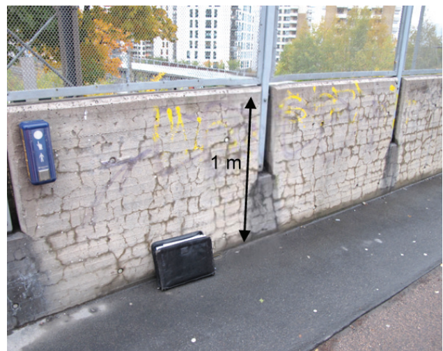
Figure 7 Visual assessment of the railing of Storo bridge, phase to the north [4]
