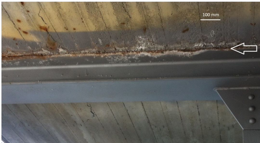
Figure 7. The saponification of alkyd paint where the painted H-beam is in contact with the concrete (marked with an arrow) and subsequent corrosion of zinc and steel.
