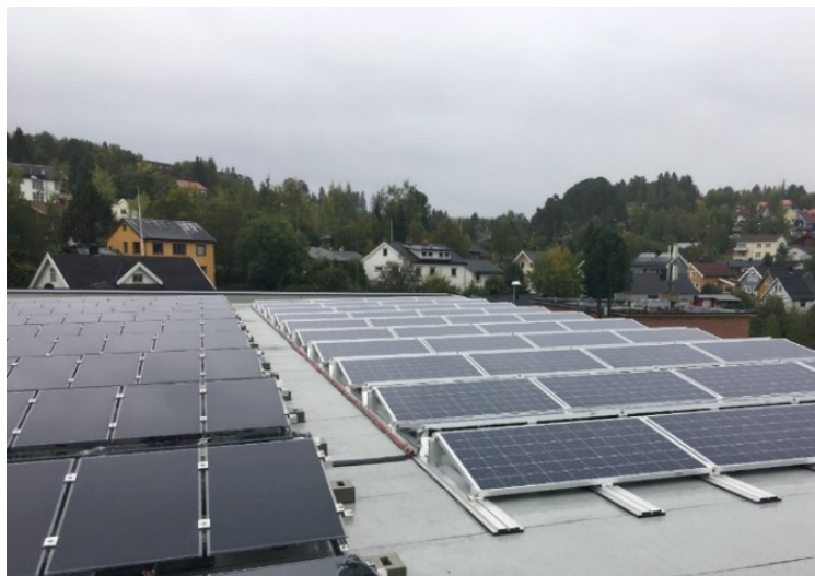
Figure 18 Solar cells on the roof of KIWI Dalgård. Left: Thin film and right: crystalline solar cells [32].
