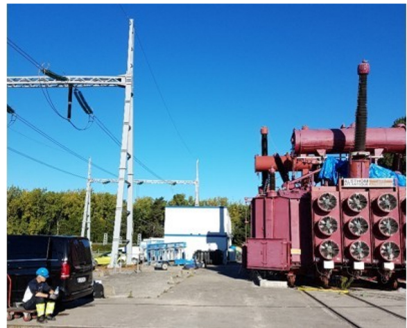
Fig. 3. HVDC 1-ph transformer measurement object.
