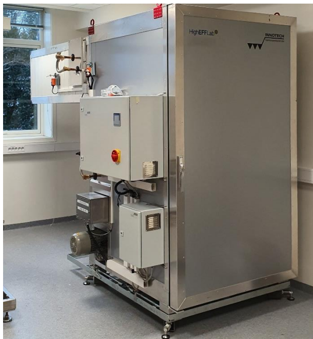
Figure 7: Installed dryer cabinet in HighEFFlab at SINTEF (including framework for weight cells).
