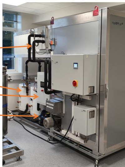
Figure 8: Heat pump fitted to the dryer (on weight cells) and ready for site acceptance tests.
