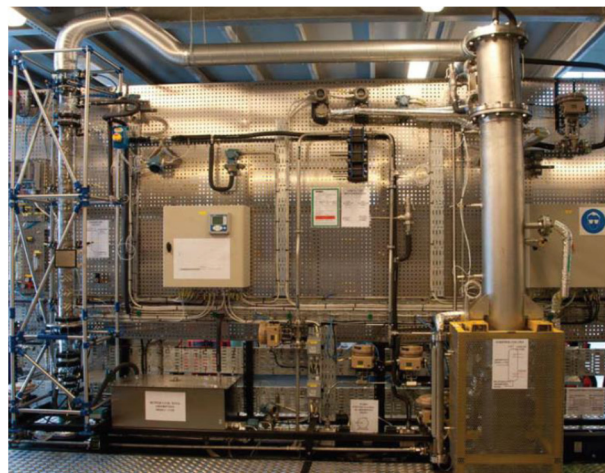
Figure 1: Amine based CO 2 capture pilot plant at USN
